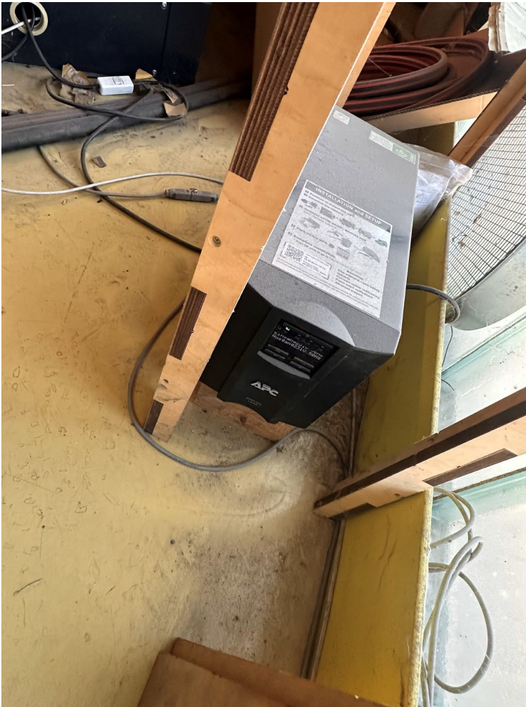
72 1 USV APC Smart-UPS 1000
