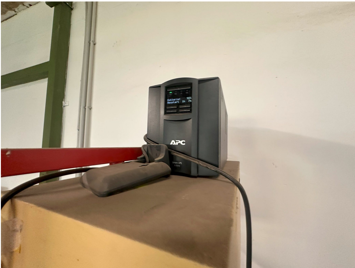
84 1 USV APC Smart-UPS 1000
